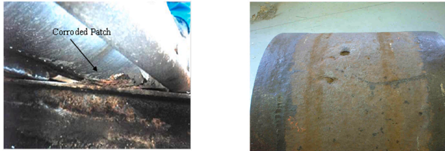
Fig. 15. Photographs of (a) corrosion at a pipe support [198]; (b) deep, highly localised pits [199].
