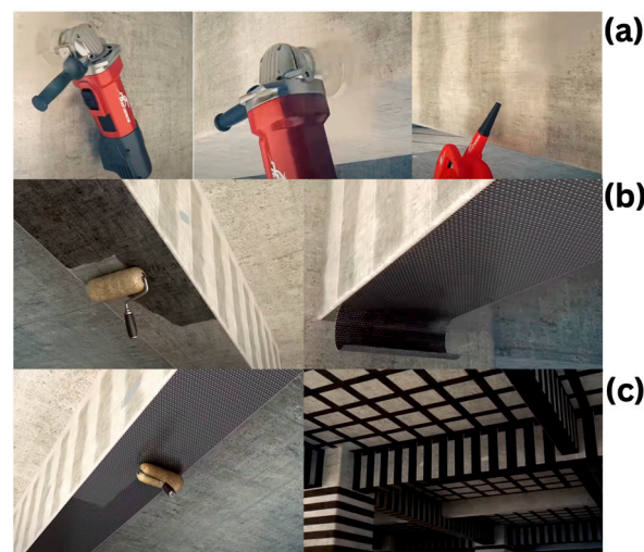
Figure 1. Application of an Externally Bonded FRP system [28]; (a) surface preparation; (b) application of resin and FRP sheets; (c) coating and finishes.
